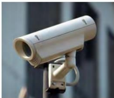
Security and Alarm Systems
